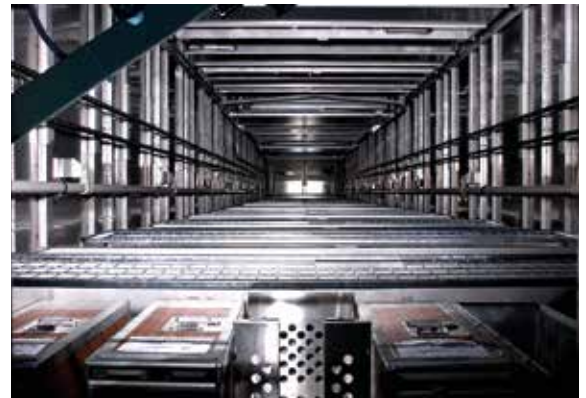
The densest trolley storage: Lödige's Space Tower
